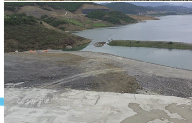
Cofferdam Over topped
